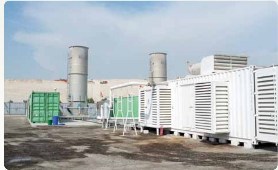
A biogas project at Al Qusais landfill site, Dubai
