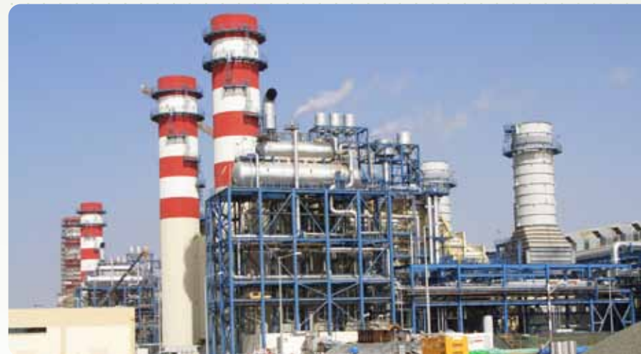
A combined cycle power plant, Abu Dhabi
